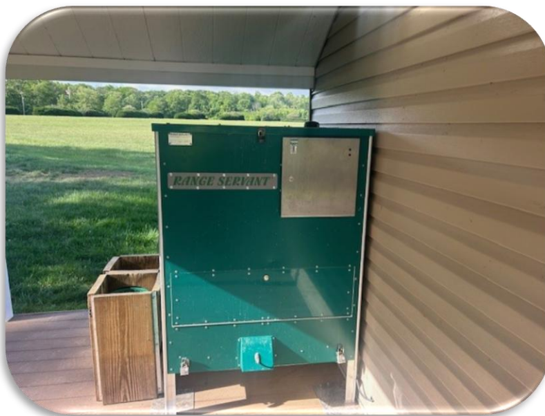
2025 public golf driving range ball dispenser, ball washer and gator were replaced.
